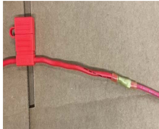
Butt Splice on Fuse Holder/+12 Volt Battery
